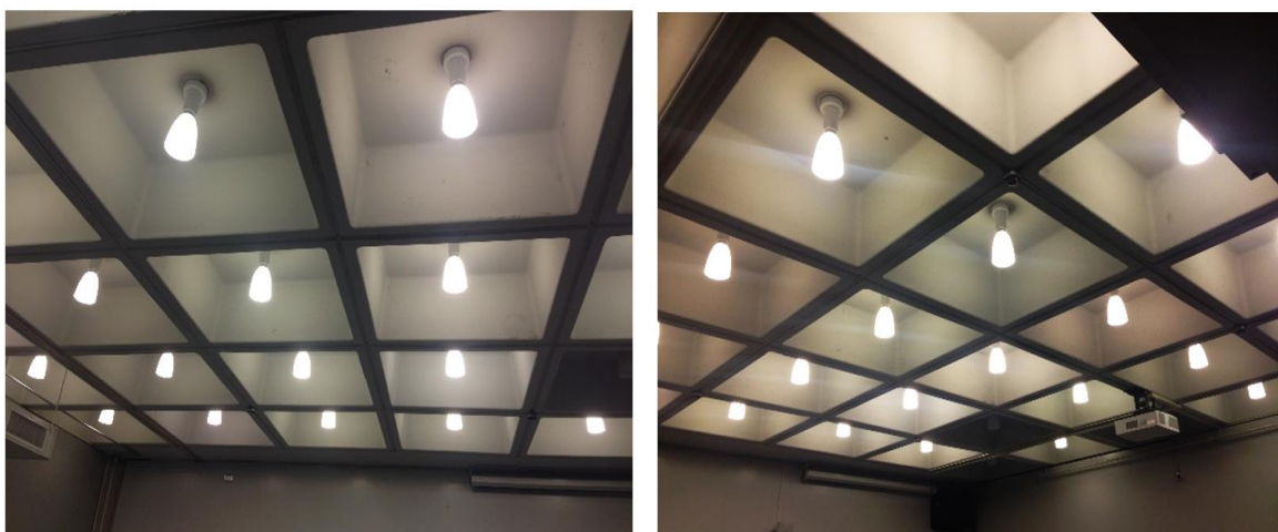
Figure 2. Shows the existing lighting arrangement in the Computer Lab
